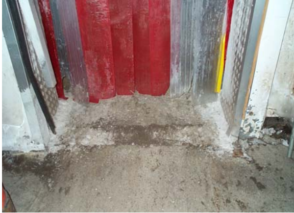
Figure 14 Iced up door and threshold before replacement
