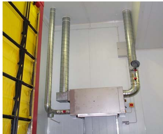
Figure 17 Wall mounted dehumidifier
