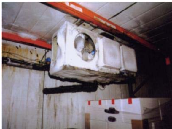
Figure 2. Iced up evaporator coil and snow-covered ceiling.
