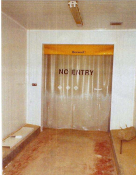
Figure 9 Air-lock in figure 7 now frost free
