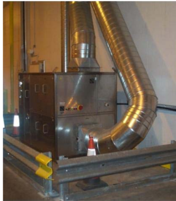
Figure 16 Large floor mounted dehumidifier
