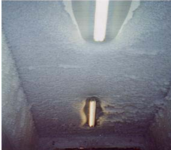
Figure 7 Frosted air-lock prior to dehumidification
