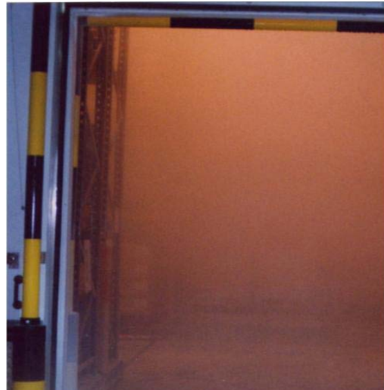
Figure 11 Entrance to a fog bound cold store
