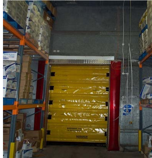
Figure 15 Cold store entrance of picture 14 after the fitting of a rapid movement door and dehumidifier.
